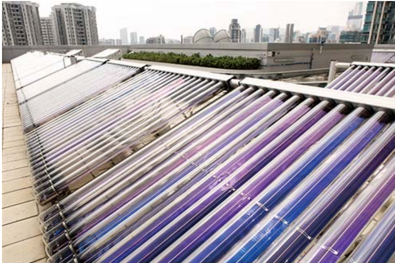
Solar panels have been installed on the roof of the Yau Ma Tei Divisional Police Station for water heating.
