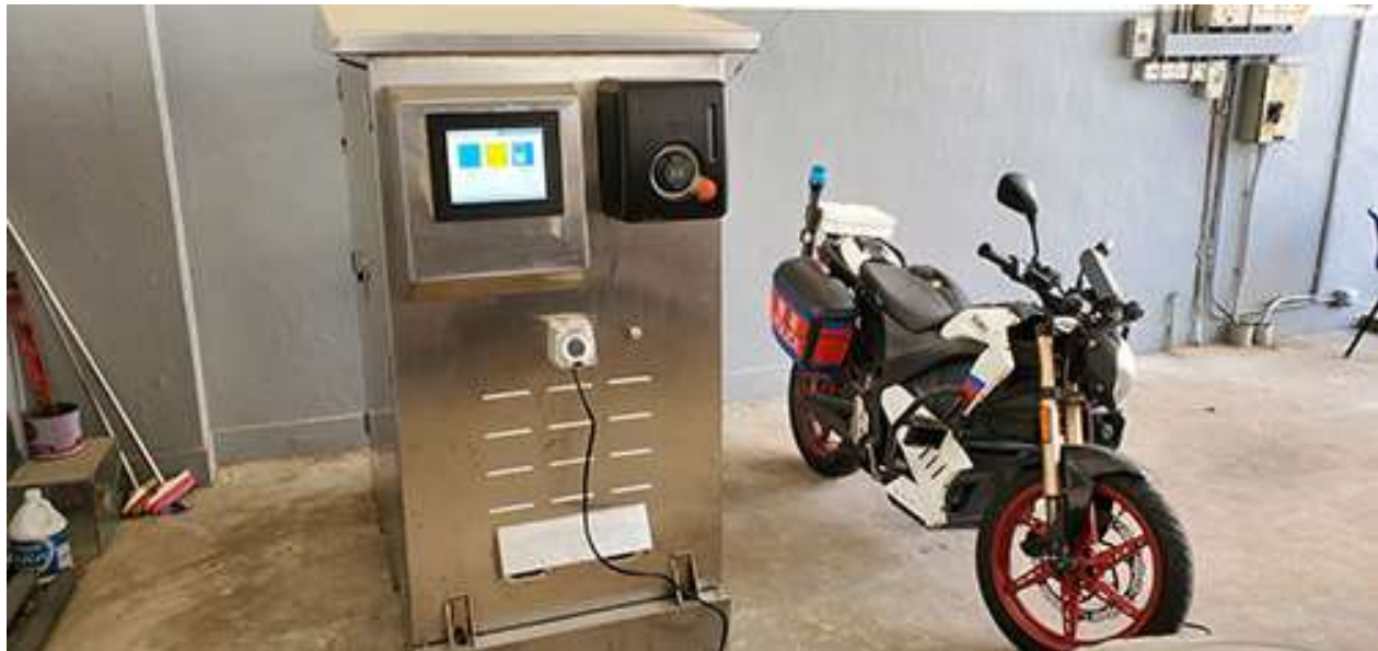
The battery storage electric vehicle station in the Police Driving and Traffic Training Centre.
