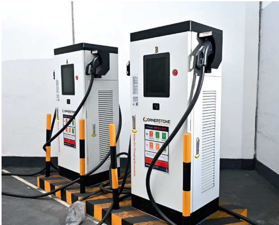
Charging points for electric vehicles at the Police Headquarters Complex.
