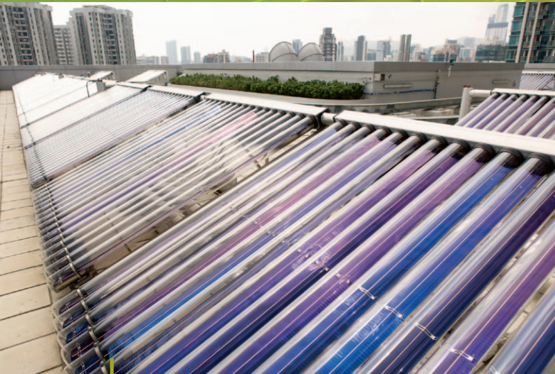
油麻地分區警署天台裝設太陽能電池板，用作加熱水溫。 Solar panels have been installed on the roof of the Yau Ma Tei Divisional Police Station for water heating.
