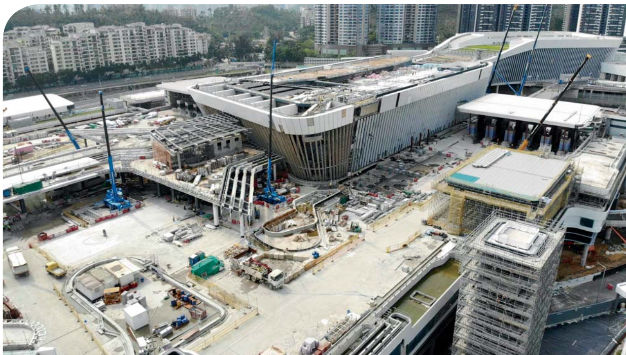
Heung Yuen Wai Boundary Control Point is under construction. 兴建中的香园围边境管制站。
