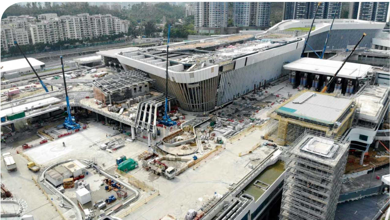
Heung Yuen Wai Boundary Control Point is under construction. 興建中的香園圍邊境管制站。
