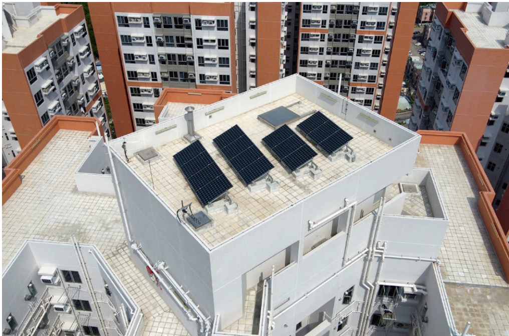
装设于芬园天台的太阳能发电光伏板。 Photovoltaic panels are installed on the roof of a residential block at Fan Garden to convert solar energy to electricity.
