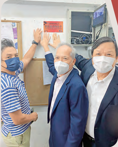
▼ DFCC members inspect CCTV system installed under NTN's "Project North-i".
